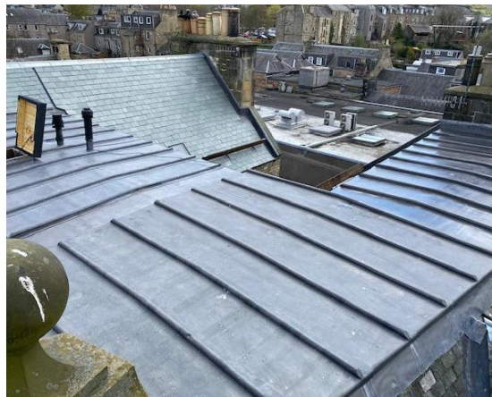
Images: Completed high level works at the former Liberal Club / 80 High Street.
