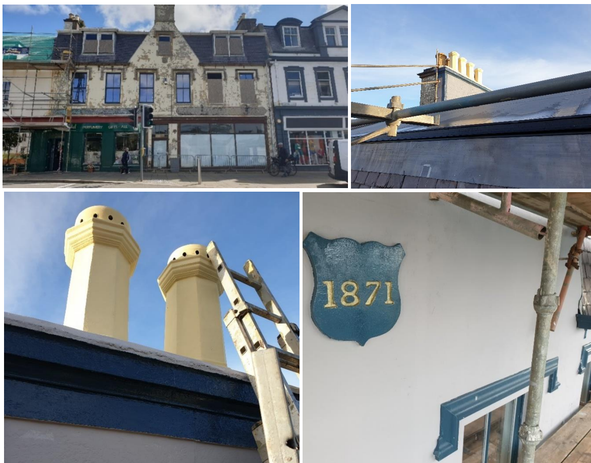
Former Murdo MacLean's, Stornoway. Top left image: before works, all other images works completed or underway.
